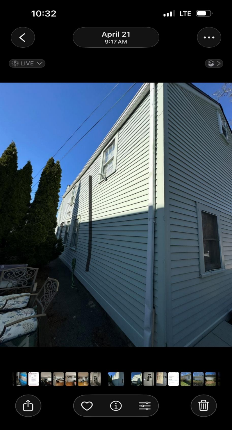
Second set of vertically run conduit lines that are not visible to the public way.
