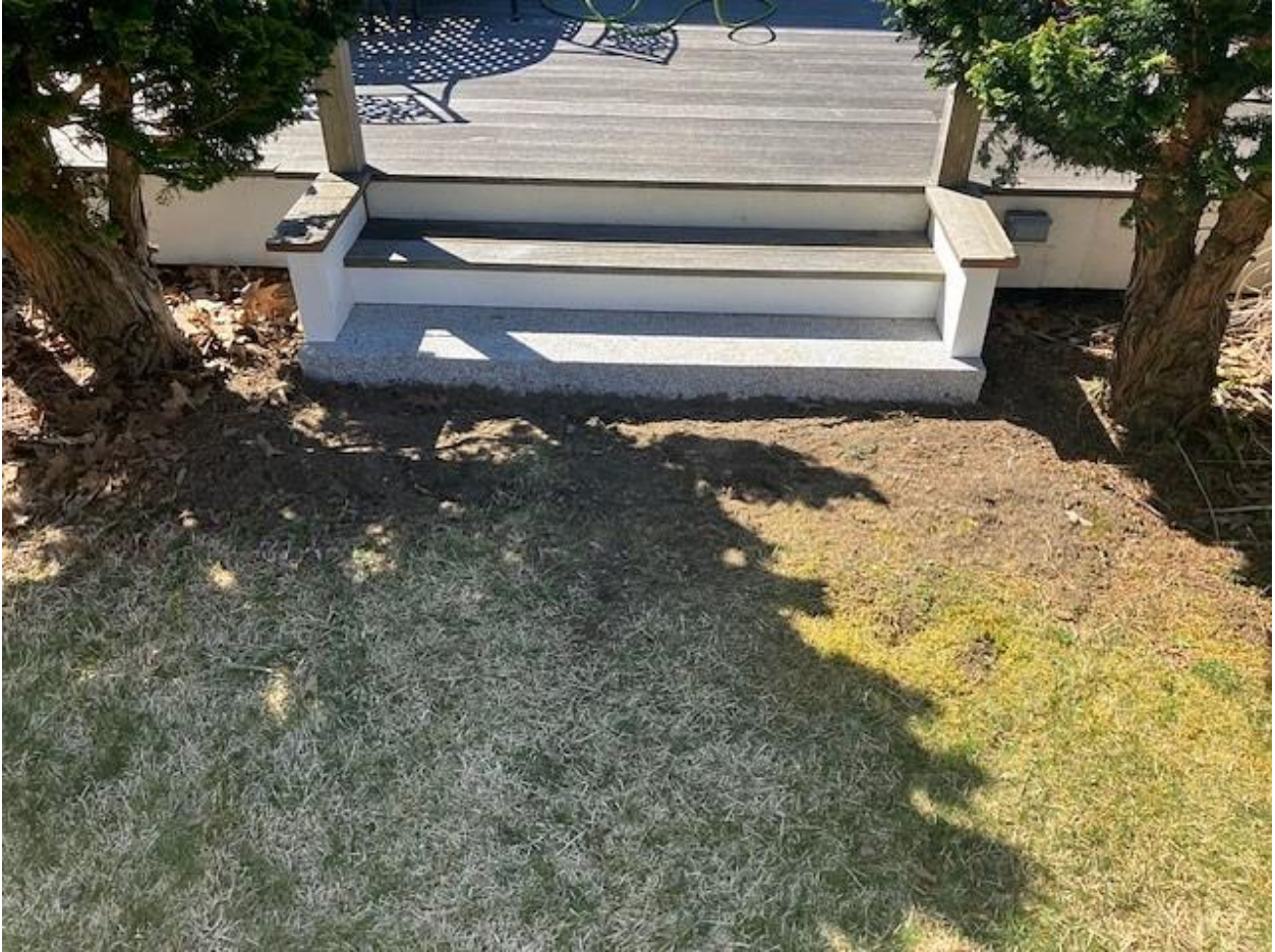
Example photo showing a granite base and composite stairs.
