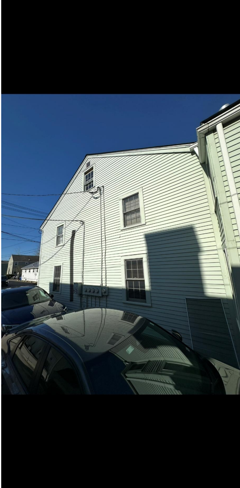
One set of vertically run conduit lines that are visible to the public way.
