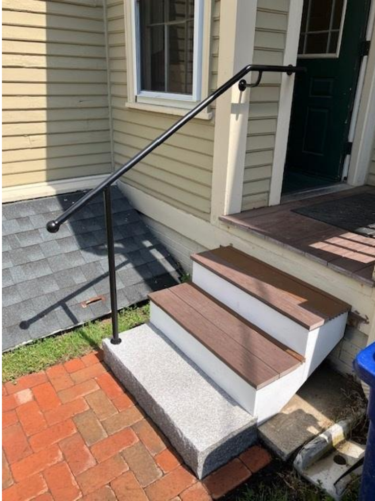
Example photo showing a granite base and composite stairs.
