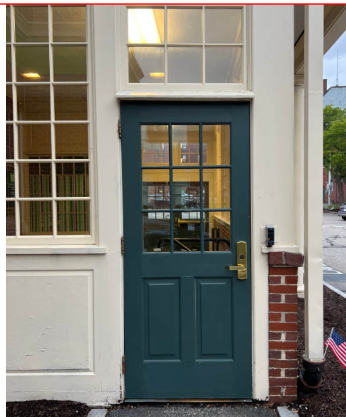
REMOVE AND REPLACE EXISTING WOOD DOOR WITH NEW ALUMINUM FACTORY PAINTED DOOR WITH 12 DIVIDED LITES. (COLOR TO BE GREEN TO MATCH EXISTING)
