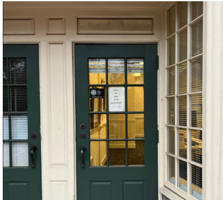
REMOVE AND REPLACE EXISTING WOOD DOOR WITH NEW ALUMINUM FACTORY PAINTED DOOR WITH 12 DIVIDED LITES. (COLOR TO BE GREEN TO MATCH EXISTING)
