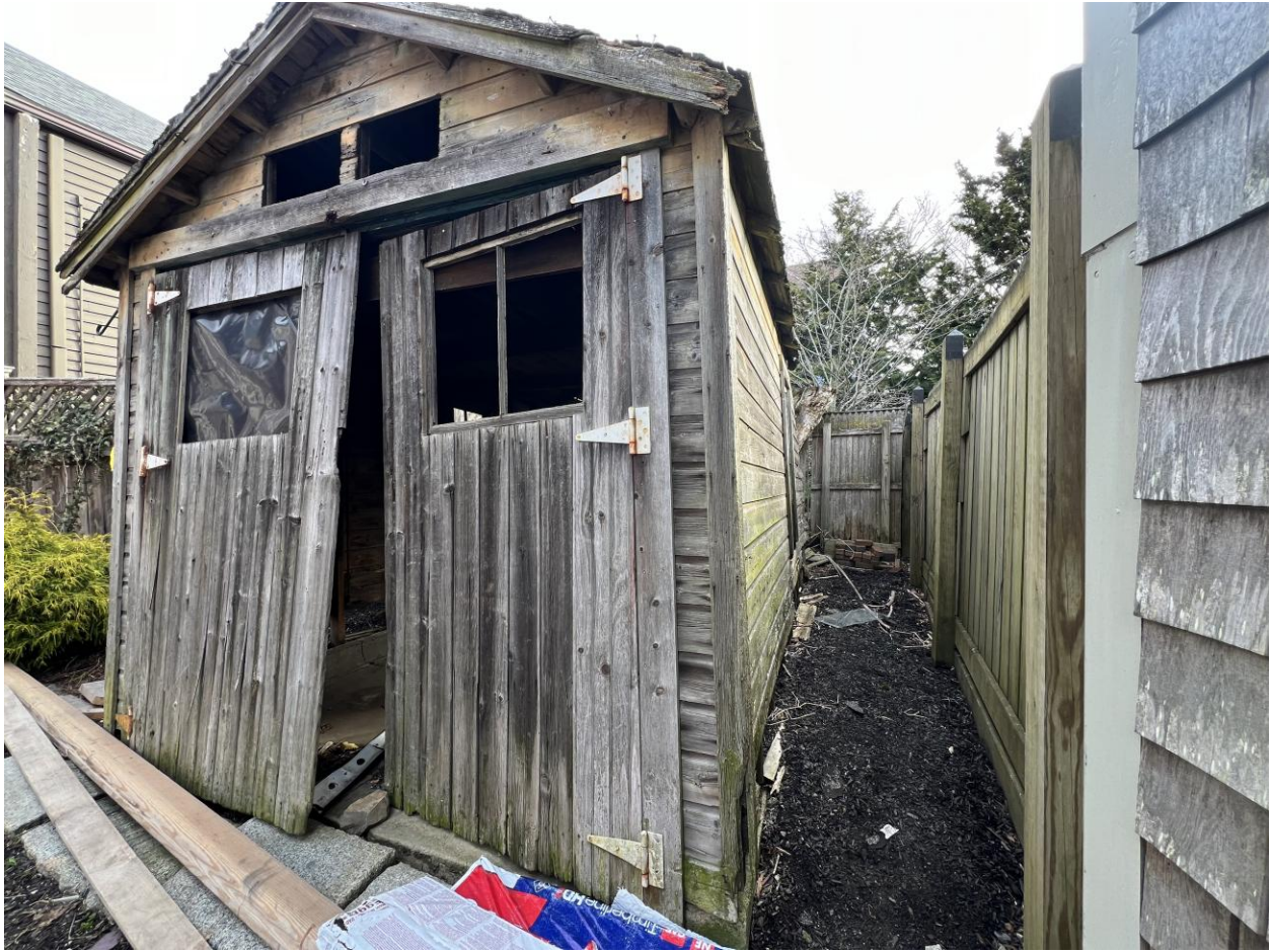
Existing shed is rotted and beyond reasonable repair.
