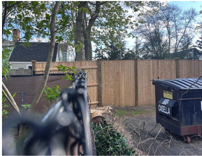
After: Photo shows new fence construction. Applicant's new fence extends to Lot 5's privacy panel. Also note, the existing dumpster's close proximity to residential properties along with the trash (artificial tree) placed against Lot 6's fence.
