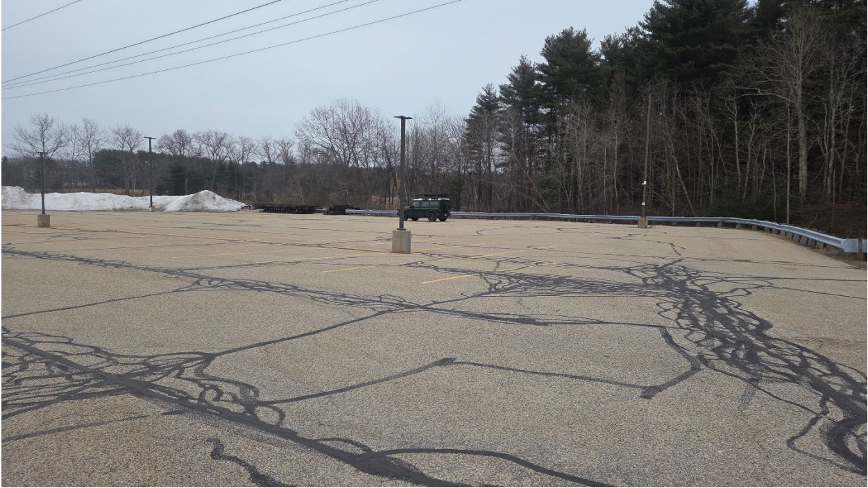
Photo 3 – Liberty Mutual – View looking southeast along the parking lot toward the Stormwater Area where impacts are proposed (Photo taken 3/20/2026).
