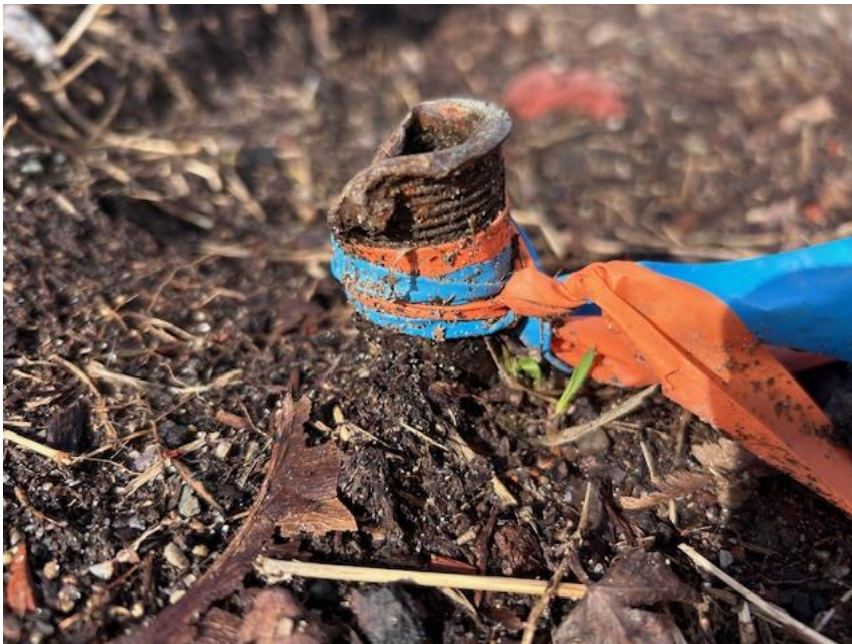
Photo shows of the 1" iron pipe is damaged and leaning. Labeled as 1" IP FOUND 0.2' Exposed on site plan survey. This is referenced as the sole marker for the eastern boundary.
