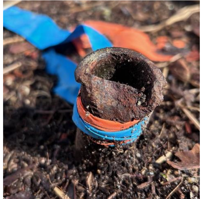
Photo shows an alternative view of the degraded and damaged condition. No additional remarks regarding damage or leaning on shown site plan survey.
