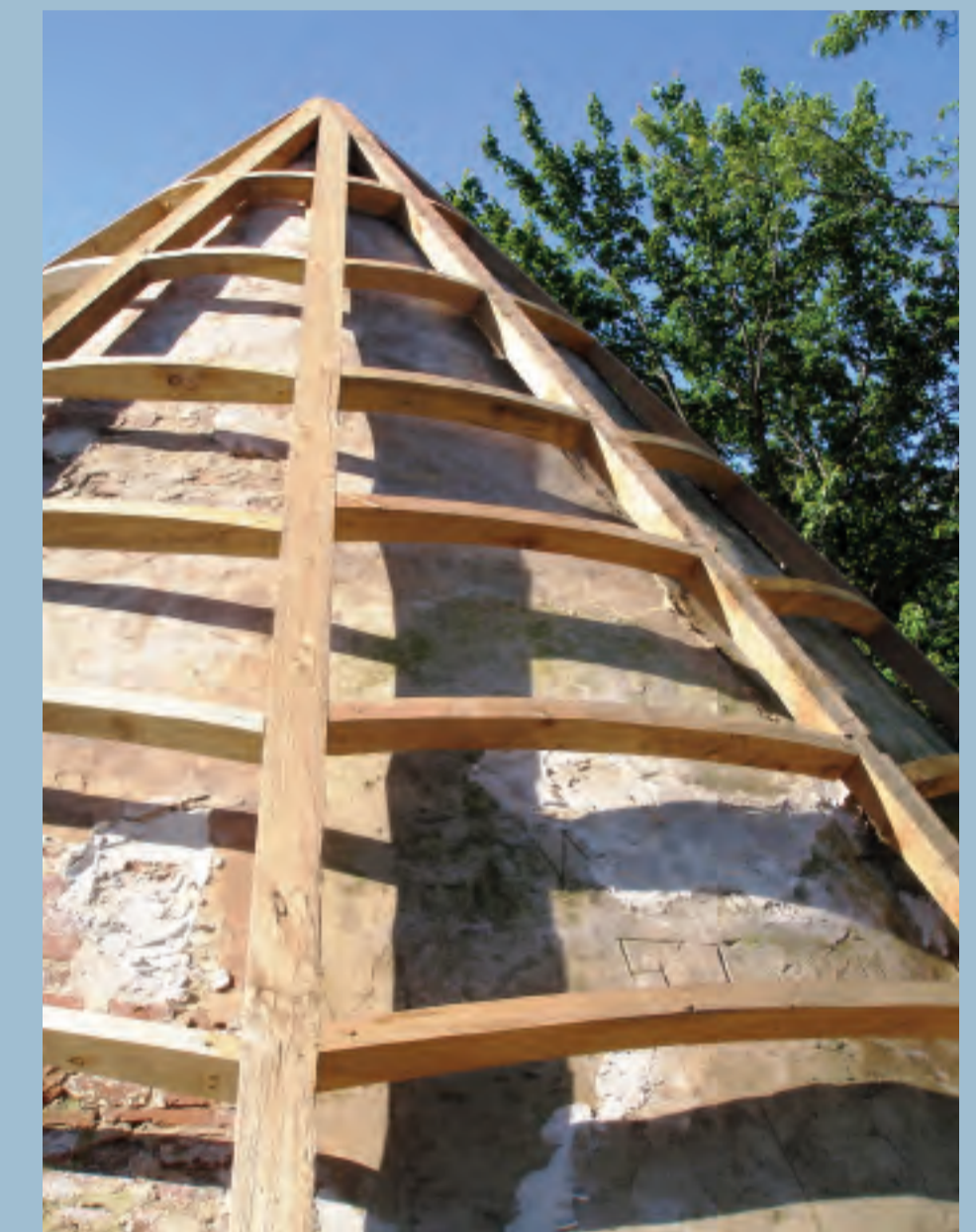
Right: Photograph of exterior work on roof showing parged roof and nailers. Above and left: Sketch from construction drawing by Susan Kress Hamilton. Courtesy of City of Portsmouth.
