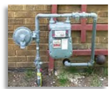
Natural gas piping
