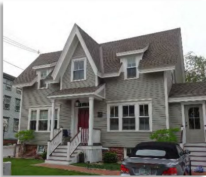
TQS/BAS/UBM Eaves cut through middle of window.
