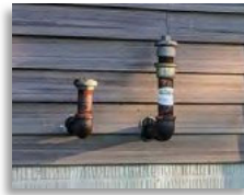
Oil tank pipes
