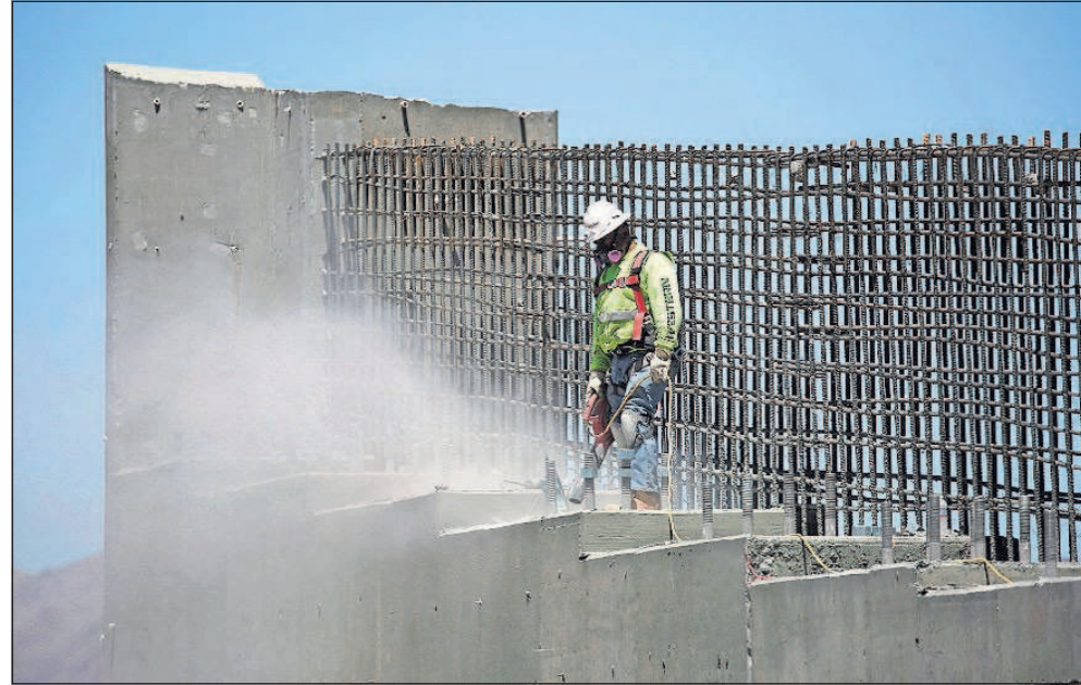
A man works on the Southern Nevada portion of U.S. Interstate 11 on May 19, 2017, near Boulder City, Nev. President Donald Trump will unveil his long-awaited infrastructure plan today, a $1.5 billion proposal that fulfills a number of campaign goals, but relies heavily on state and local governments to produce much of the funding. [JOHN LOCHER/THE ASSOCIATED PRESS, FILE]
