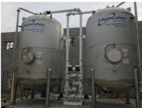
New Granular Activated Carbon (GAC) Filters
