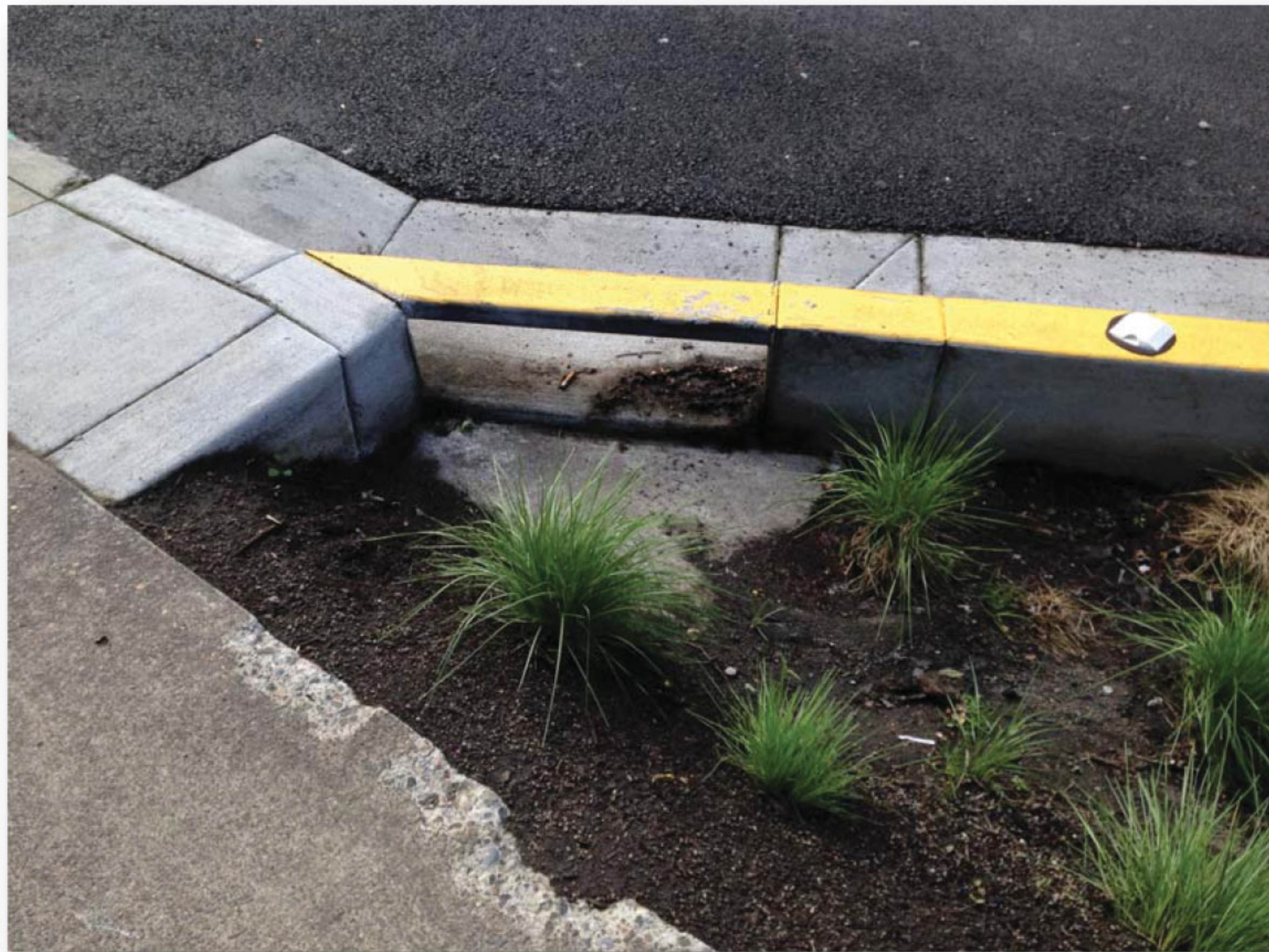
Curb cut inlet allows stormwater to enter the stormwater planters for infiltration, filtering, and plant growth before entering the stormwater system.
