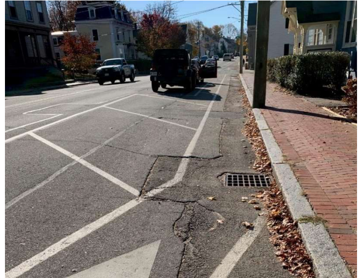
Figure 1: Photo of pavement seam and catch basin at start of southbound bike lane, and parked car with open door visible
