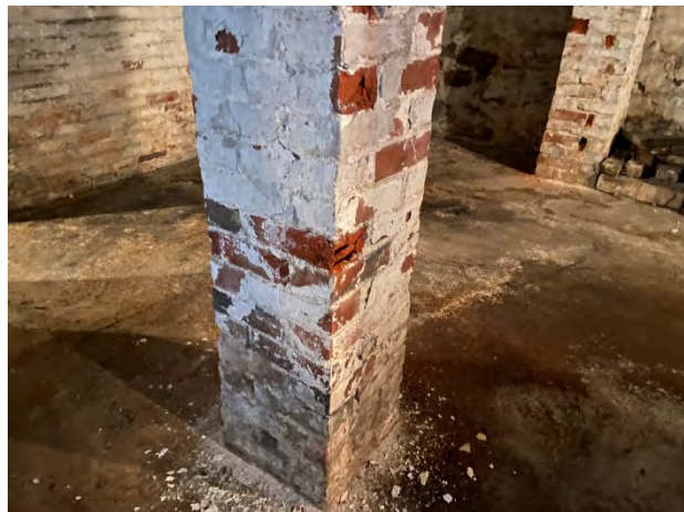
6 - Masonry pier deterioration
