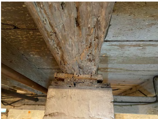
9 – Decayed timber on masonry pier
