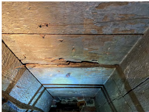
10 – Area of decayed floor deck
