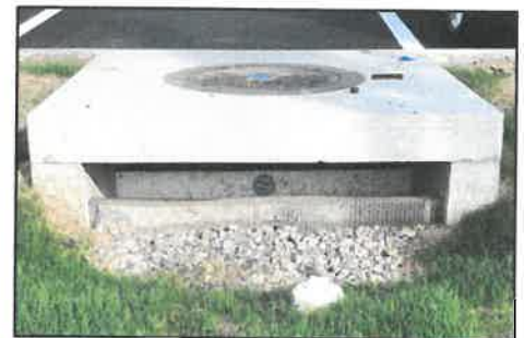
REAR VIEW OF OUTLET SCREEN
