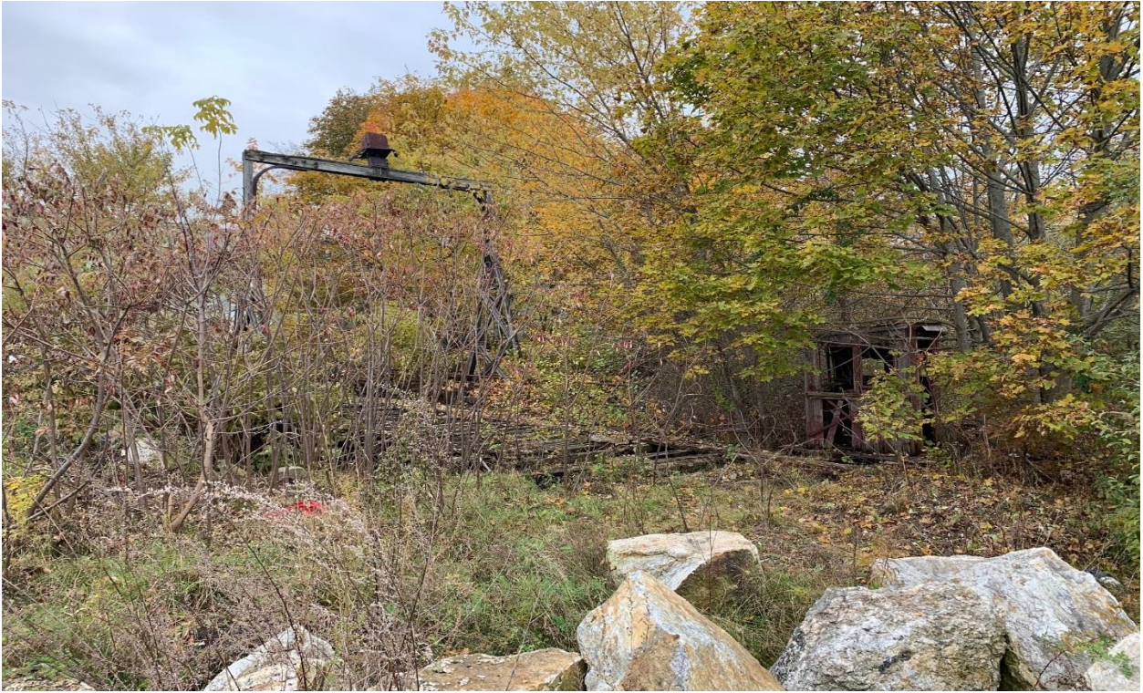
Limited ground cover removal needed to access turntable for demolition. Access via existing pavement.
