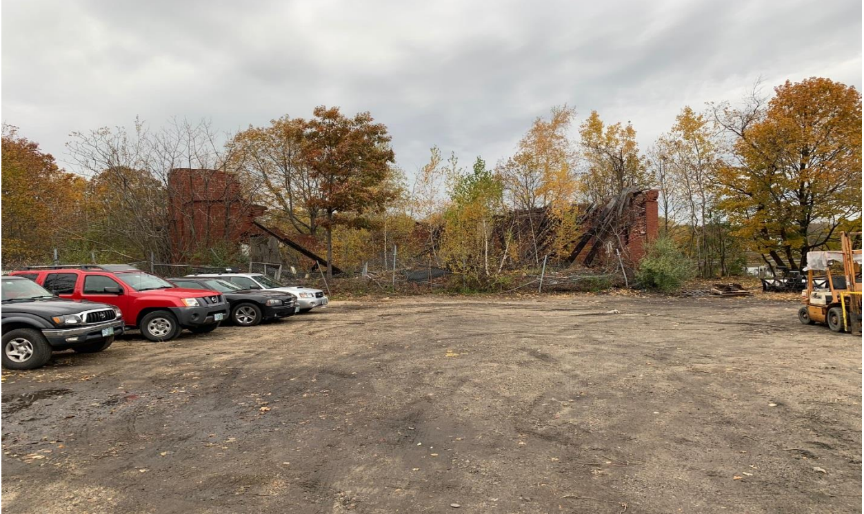
Access to structure for demolition via existing parking lot. Some trees growing within structure footprint.
