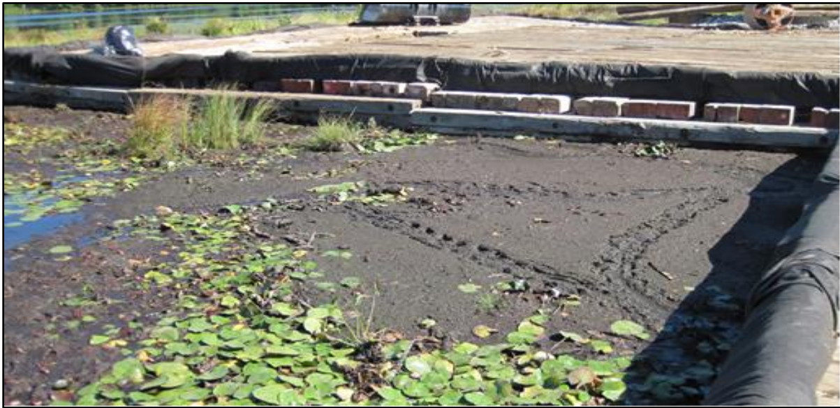
Location showing impeded aquatic organism passage due to swamp matting placement.
