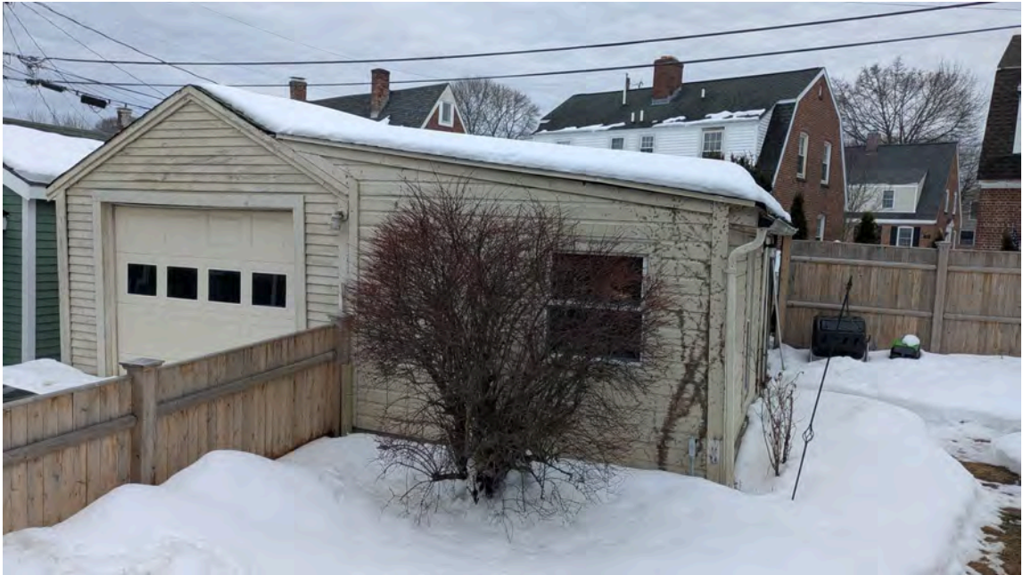
PHOTO 4: FRONT VIEW OF GARAGE, GARAGE OPENING SHOWING VISIBLE SIGNS OF STRUCTURAL RACKING
