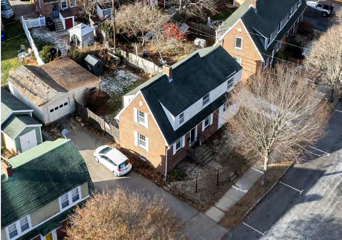
PHOTO 1: AERIAL VIEW OF PROPERTY. GARAGE ROOF AT END OF LIFE
