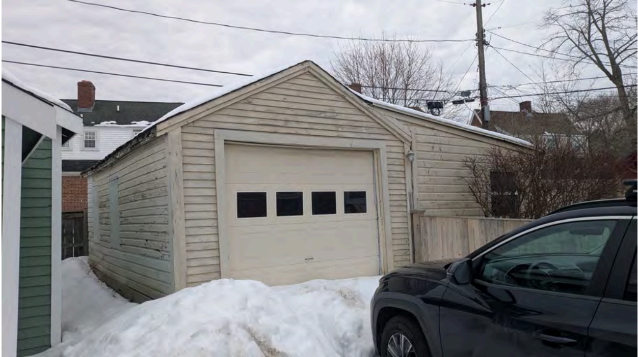
PHOTO 5: FRONT VIEW OF GARAGE, GARAGE OPENING SHOWING VISIBLE SIGNS OF STRUCTURAL RACKING. ROTTED SIDING & TRIM
