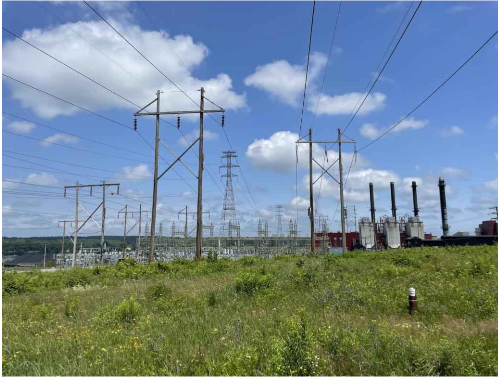
Photograph No. 21: Looking northeast at Structure 1 on the T13 Line ROW off Gosling Road, Portsmouth, NH.
