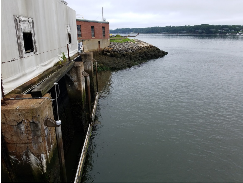
Photo 4. View of units 6, 5, and 4, facing northwest (east of intakes, intake hoses for test screens will enter at unit 4)
