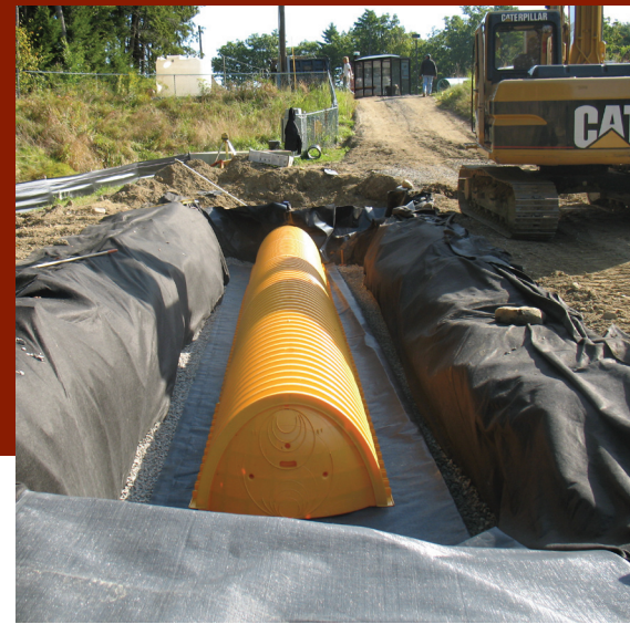
StormTech Isolator Row.
