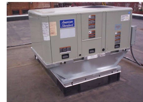
ROOF TOP UNIT
