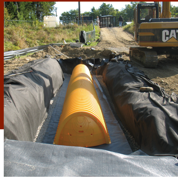
StormTech Isolator Row.
