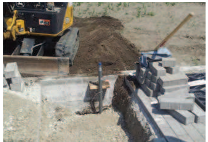
Backfill and ensure riser is set correctly. Conclusions of the Enbridge Gas exercise
