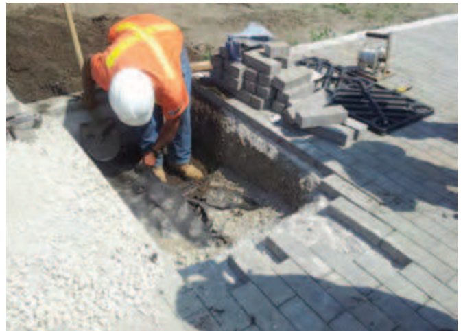
Cover over the cell deck with the cut geotextile and add an overlapping layer of geotextile on top.
