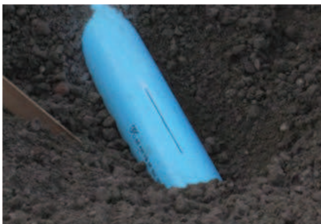
Water pipe cut.
