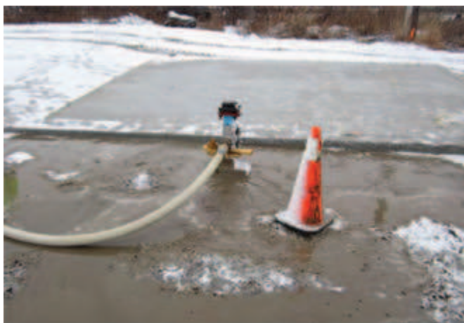
Water introduced - water bursting out of saturated soil adjacent to installation.
