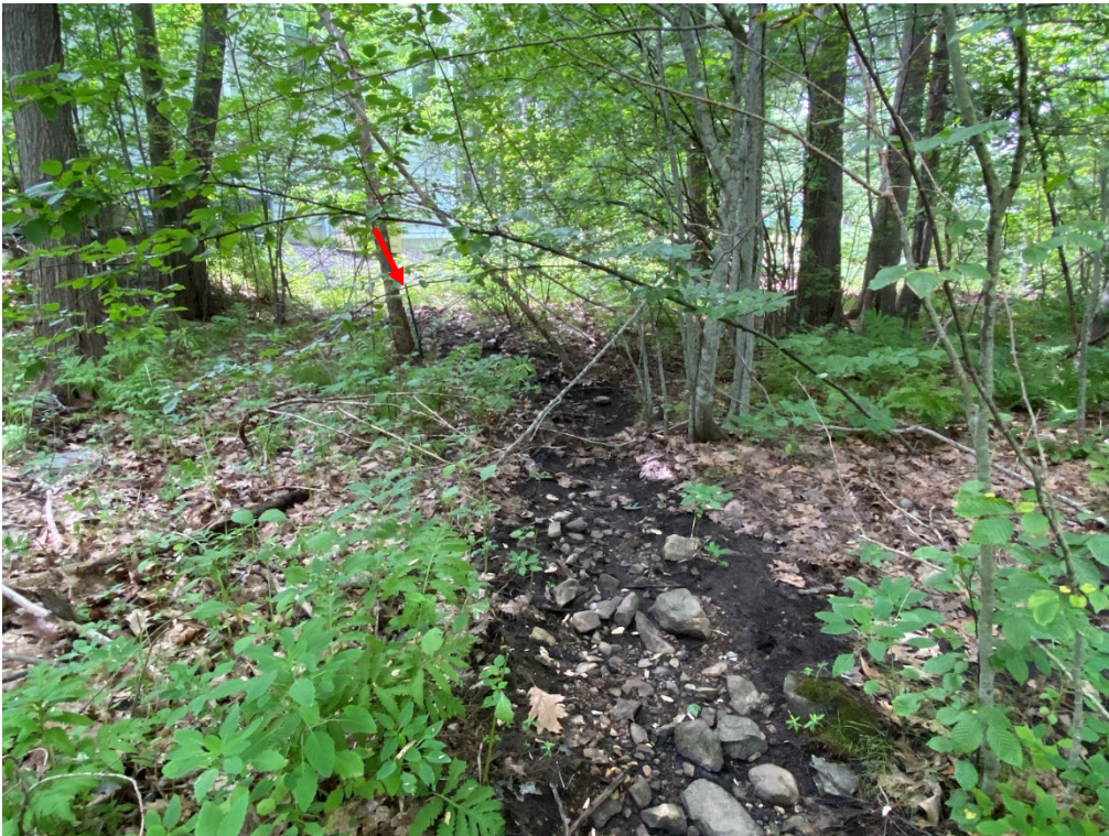
Photo 20. POGS1 leading onto the Gardner property from the culverts located at the northeastern end of POGW2, viewing south, downstream. Property boundary is indicated by the green rod indicated by the red arrow. (08-11-22)
