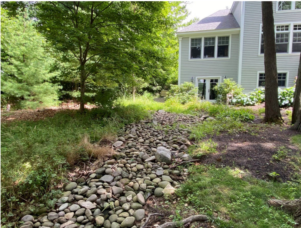
Photo 28. Overview of the older, upper portion of the stone swale, viewing east upslope. (08-11-22)
