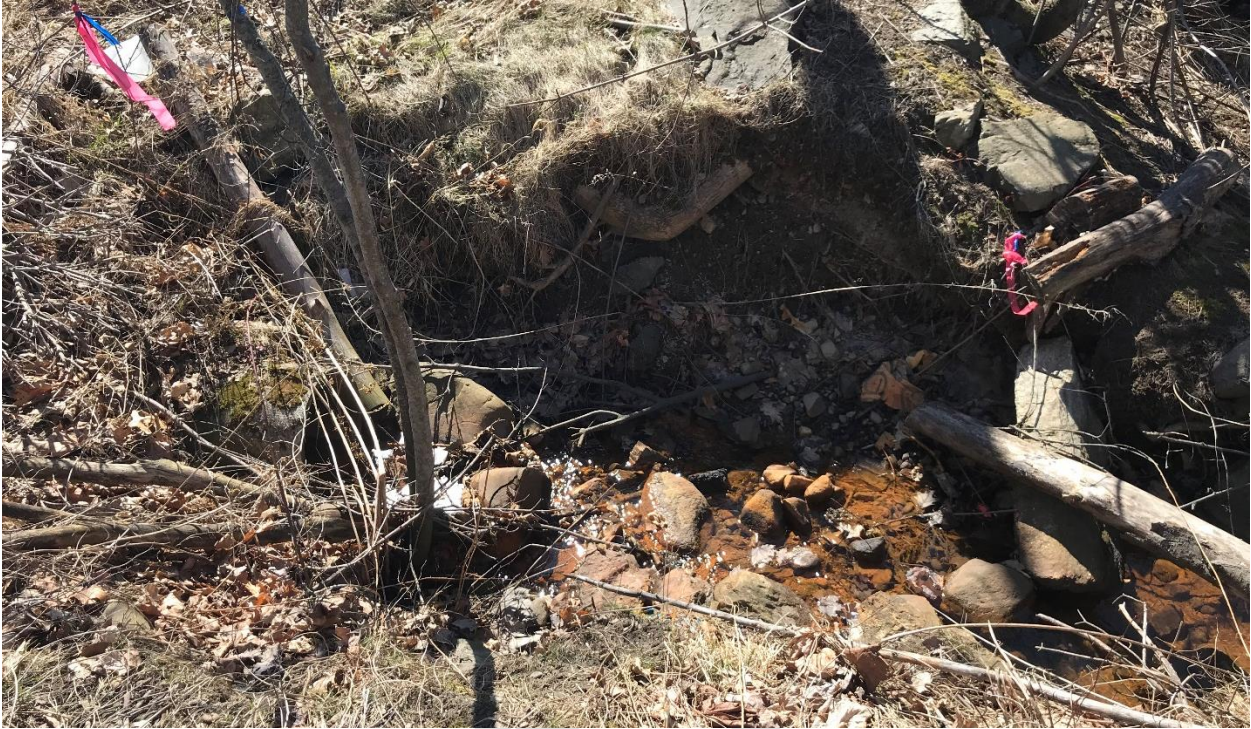
Photo #9: Looking at the area near Route 1 where the culvert area has eroded a large area.
