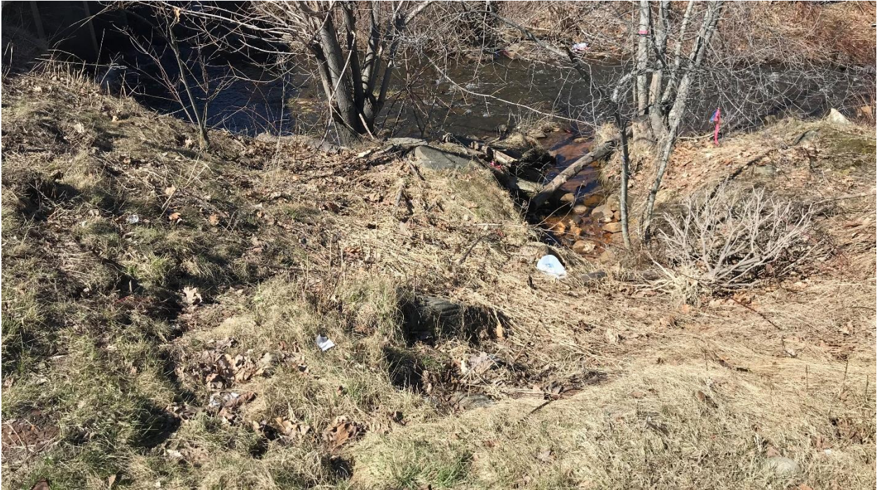
Photo #10: Looking from the top of the bank down to the area eroded by the culvert also noting that storm water runoff is starting to erode above the culvert.
