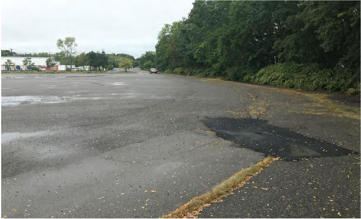
Photo #05: Looking out at the the open lot area to the intersection of Borthwick Ave and Route 1
