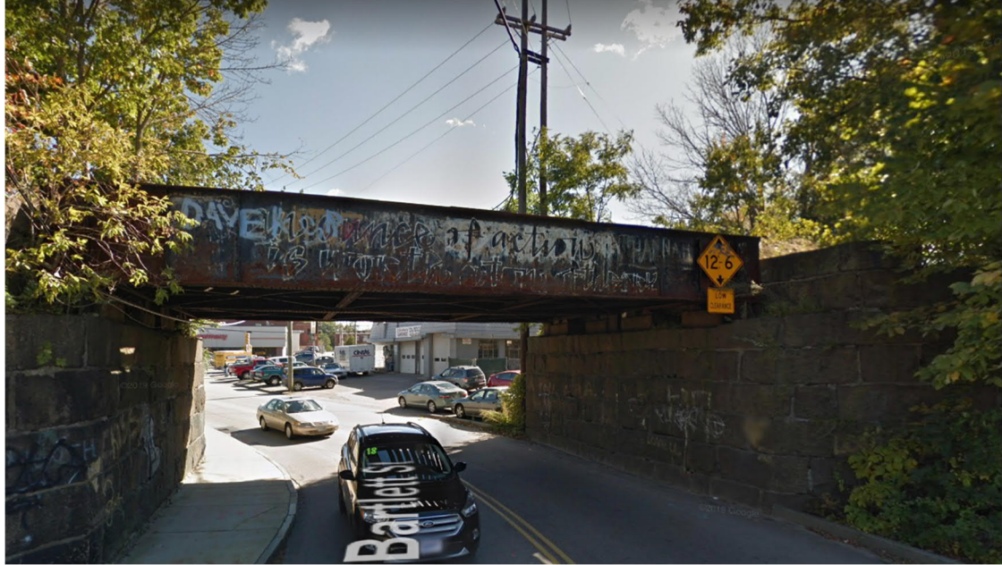
Bartlett Street looking south through the railroad overpass toward Islington Street – Low Clearance 12'6"
