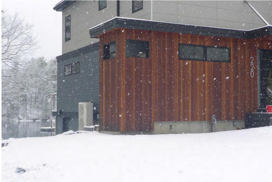
Photo 13: Facing south at 220 Walker Bungalow Road. Proposed location of piping and grinder pump in existing maintained lawn within the 100' TBZ and 75' salt marsh setback. Sagamore Creek is seen on the left and salt marsh is at the toe of slope.
