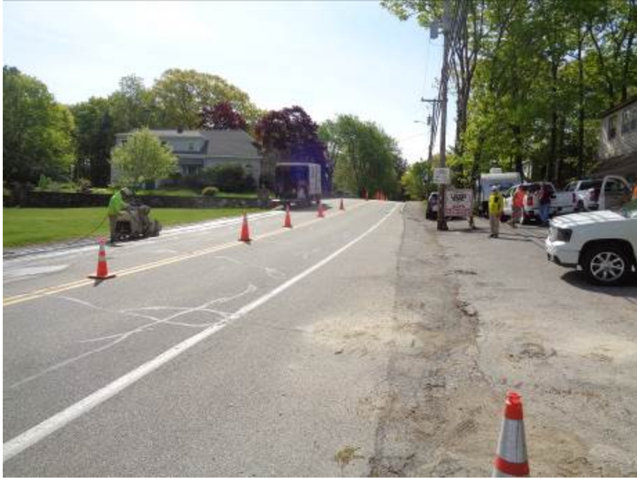
Street Scene - Front of the Subject Property Looking Southeast on Sagamore Avenue - (5/22)
