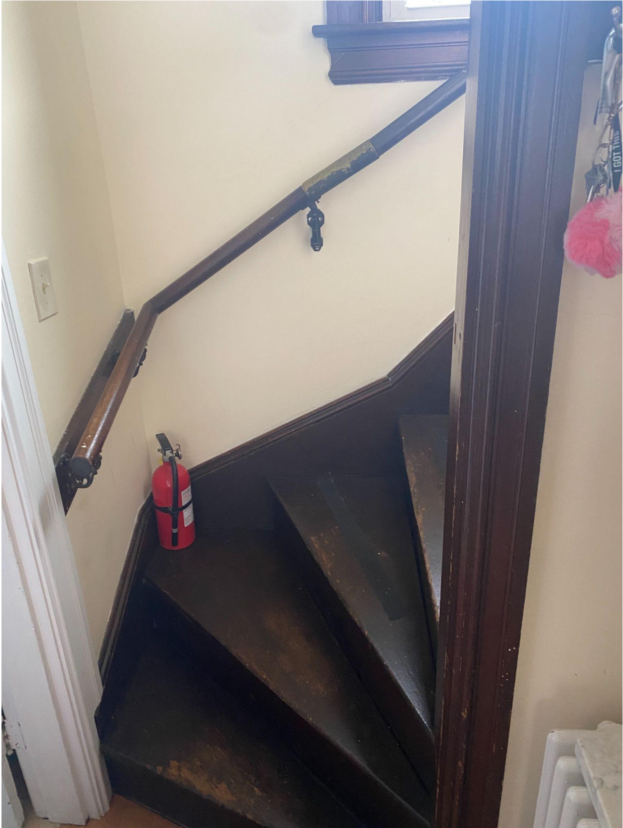
Existing Back Stairwell (Steep/Not to code)
