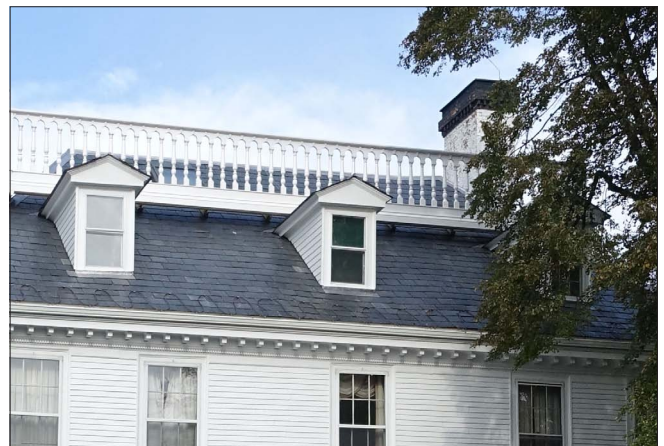
The roof, balustrade and cornice were replaced using compatible materials, that convey an appearance that is similar to the historic condition prior to storm damage.
