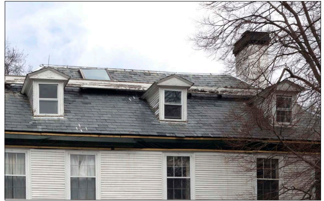
The roof surface, balustrade and cornice were damaged by heavy snow and were replaced to match the historic conditions. (Refer to photograph below.)
