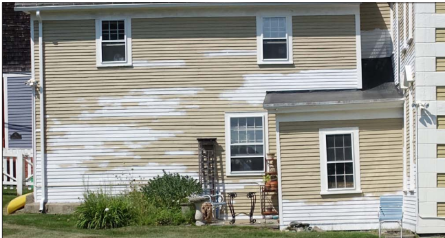
Regular repainting with proper preparation is one of the best ways to maintain exterior woodwork and siding.
