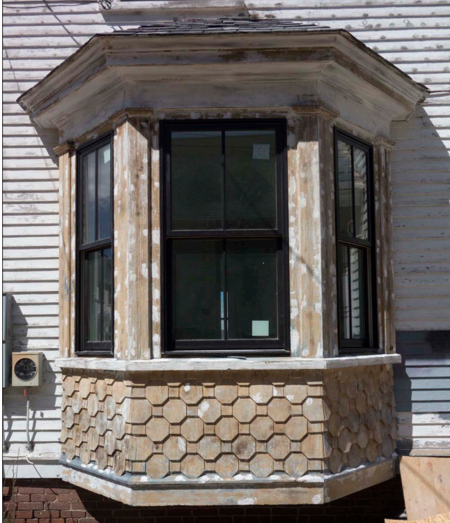
Repainting should be considered as part of regular exterior maintenance as a means of protecting wood from exposure to the elements and moisture-related deterioration.
