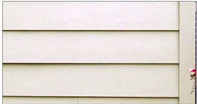
Fiber-cement siding and trim generally does not have the same dimensions as traditional wood elements including the width of corner boards and the depth of individual clapboards. This results in a visual difference, including shadow lines, as compared to wood siding.
