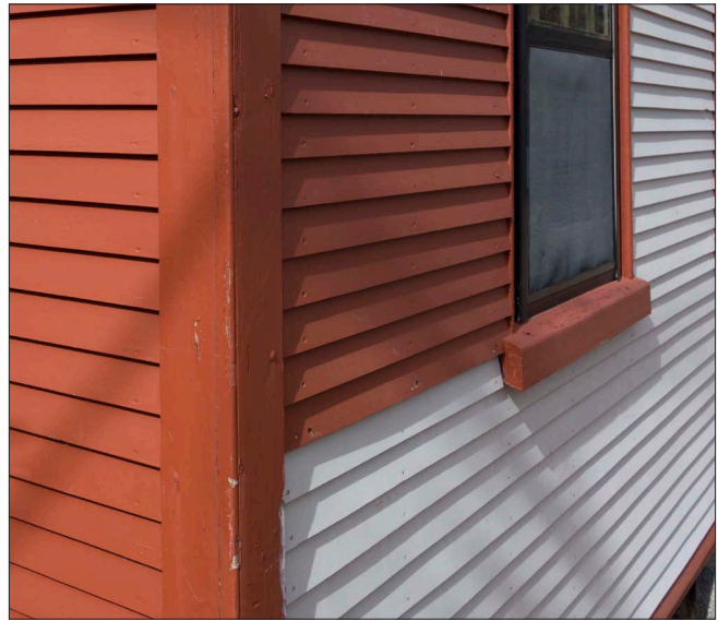
The application of a quality wood primer and two coats of paint can minimize the potential for wood rot. Note the alignment of the siding with the bottom of the window sill.
