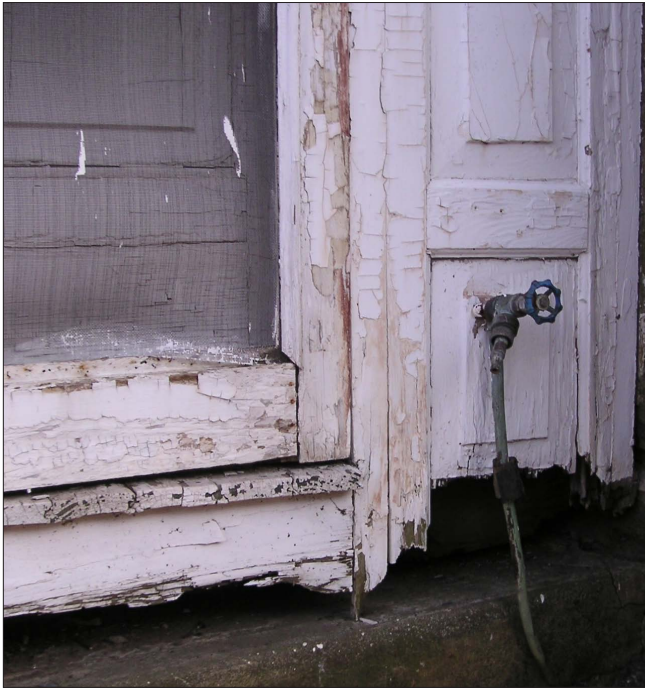
Leaking plumbing, including exterior hose bibs, can regularly expose woodwork to moisture, eventually resulting in rot. Wet wood can also be a desirable home for pests such as termites.
