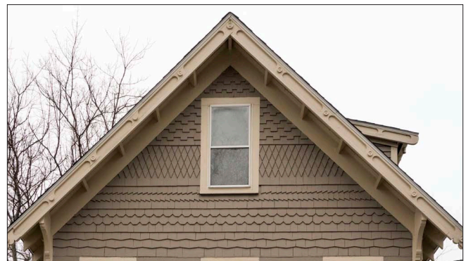
Victorian-era buildings often include a variety of shingle shapes as a decorative feature at gable ends. Note the ornate rake boards.
