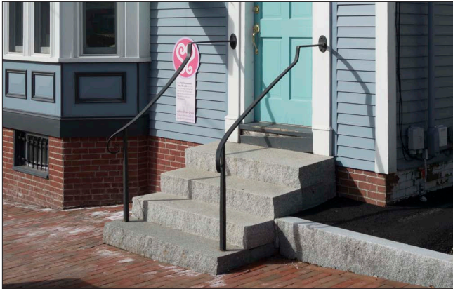
A simple, unobtrusive, metal rail was added to the granite steps to provide secure access to the door.
