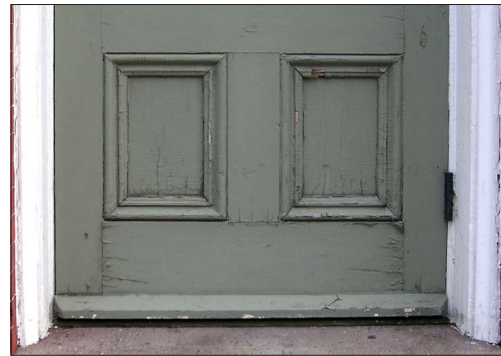
Wood checking and peeling paint is visible. Minor repair and maintenance can prolong the serviceable life of this door.
