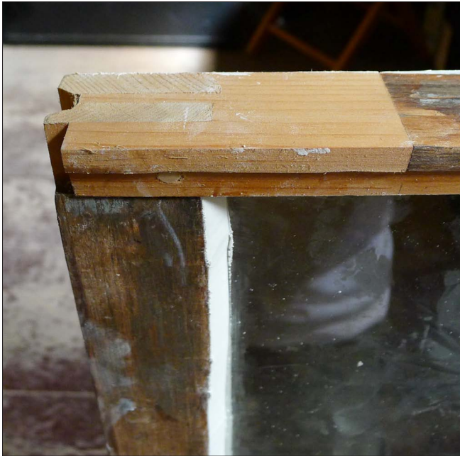
One of the advantages of historic wood windows over a modern prefabricated unit is repairability. This photograph demonstrates a Dutchman repair at the corner of the historic wood window sash. Also note the application of new glazing putty as part of the repair.
