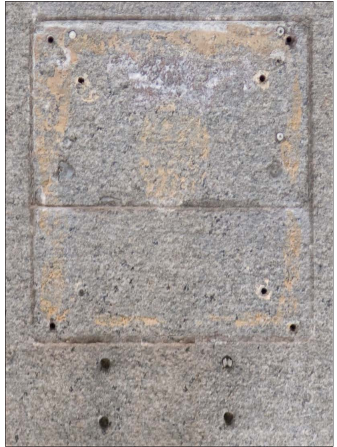
Numerous holes have been drilled into the face of the granite and several fasteners still remain. Existing holes should be reused for future signs, and abandoned holes should be filled and the stone surface cleaned. (Refer to Guidelines for Masonry & Stucco .)
