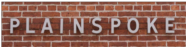
When installing pin-mounted signs in masonry, fasteners should be installed in mortar joints rather than in the face of brick or stone units whenever possible.
