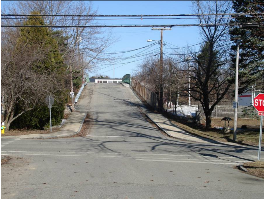
Today, the Stark Street bridge has narrow sidewalks that are not contiguous with the Dennett Street intersection and are in poor condition.
