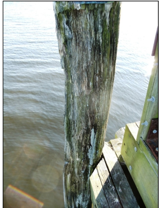
Photo 8: Typical deteriorated fender pile on South Pier
