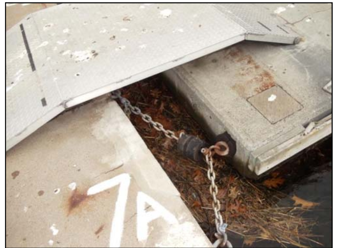
Photo 4: Temporary repair to float module connection at T-head
