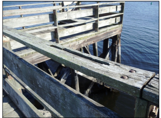
Photo 6: Typical Fungal Decay on Railing
