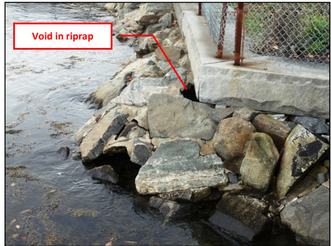
Photo 14: Void in riprap at South Pier abutment
