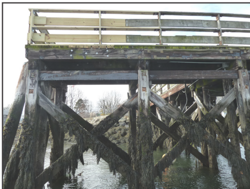
11. T-Head pier Recent repair from arson event. It is estimated that the T-Head Pier has 20 years of service life remaining, assuming it is repaired and maintained.
