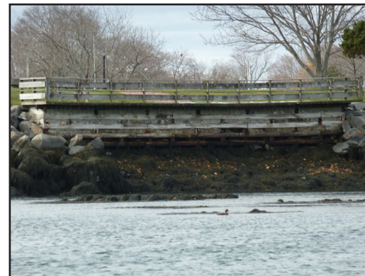
24. Four Tree Island Deck with missing rip rap and erosion undermining structure along east shore.
