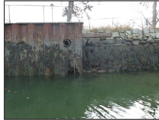
20. Steel bulkhead Significant settlement and slumping visible. Wall requires reconstruction.
