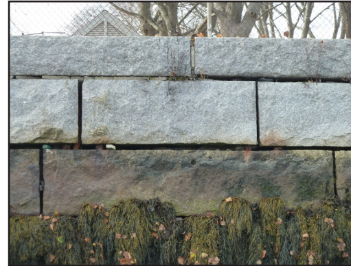
14. Quaywall Repoint and mortar joints.
