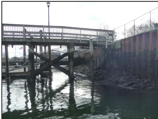
21. North Pier It is recommended to replace the timber bracing as soon as possible.
