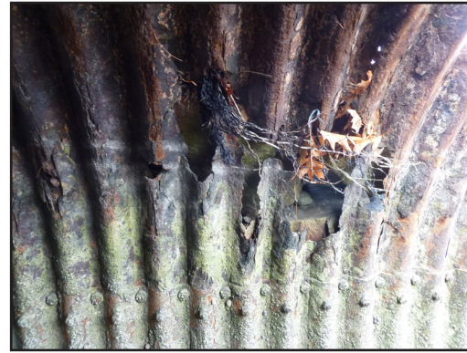
26. Four Tree Island Culvert under causeway requires lining or reinforcement. Excessive section loss in areas.
