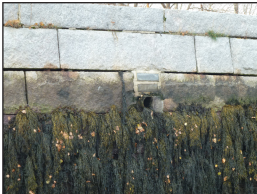
15. Quaywall Stromwater out fall.
