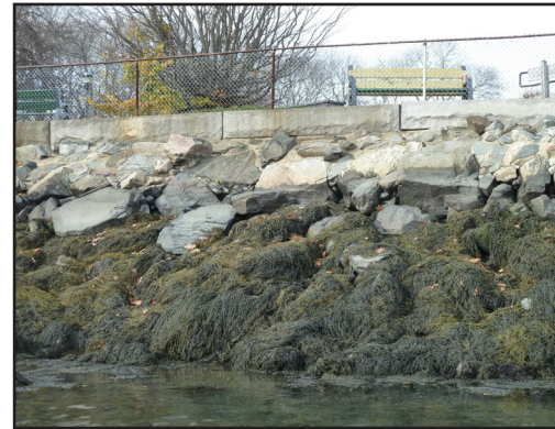
10. T-Head pier Slumping rip rap in front of set granite blocks.
