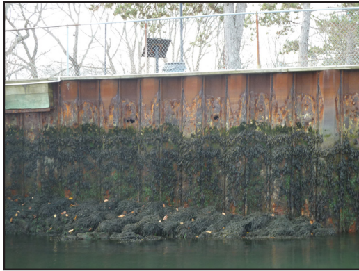
19. At north pier Steel is deteriorating with significant pitting with visible holes at high tide line.
