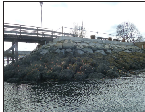
12. T-Head pier Sloped placed rip rap, top course to be reset.
