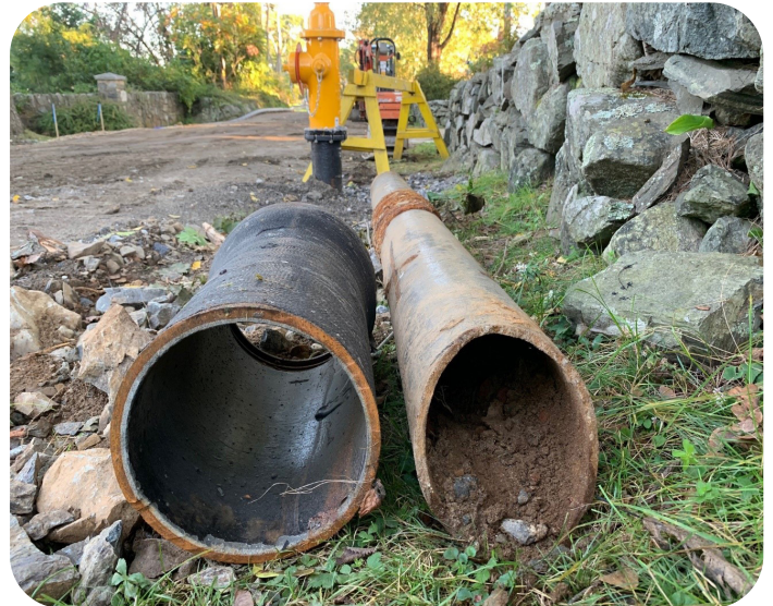
Wild Rose Lane Waterline Replacement Project New 8-inch ductile iron pipe next to old 6-inch cast iron pipe
