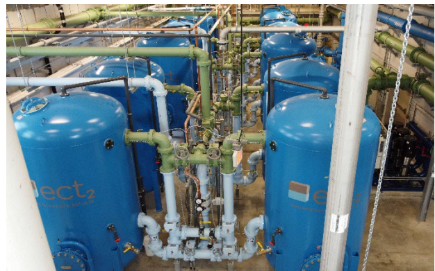
Ion-Exchange Resin Filters
