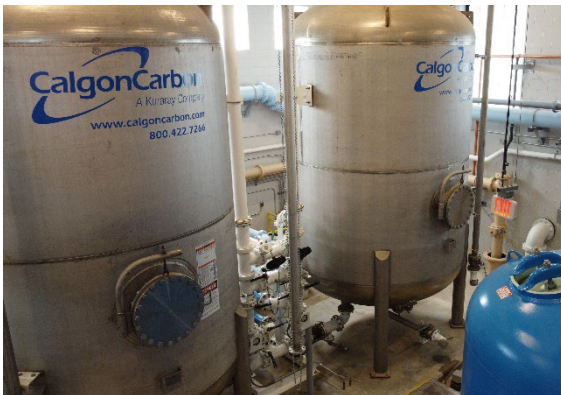
Granular Activated Carbon (GAC) Filters
