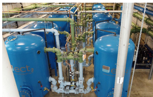
Ion-Exchange Resin Filters
