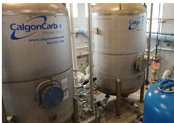
Granular Activated Carbon (GAC) Filters
