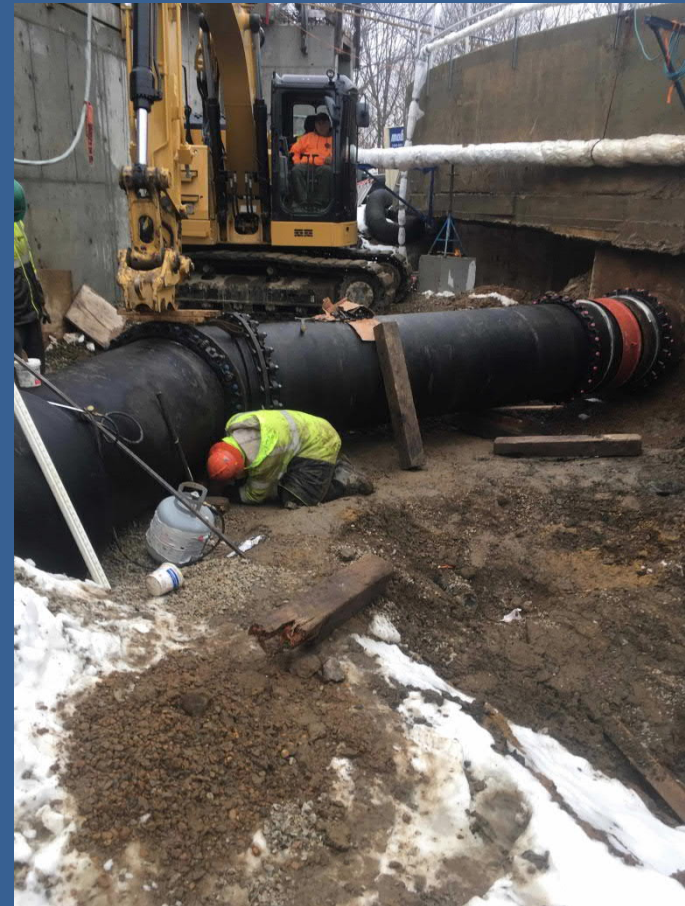
Yard Piping & Utilities
