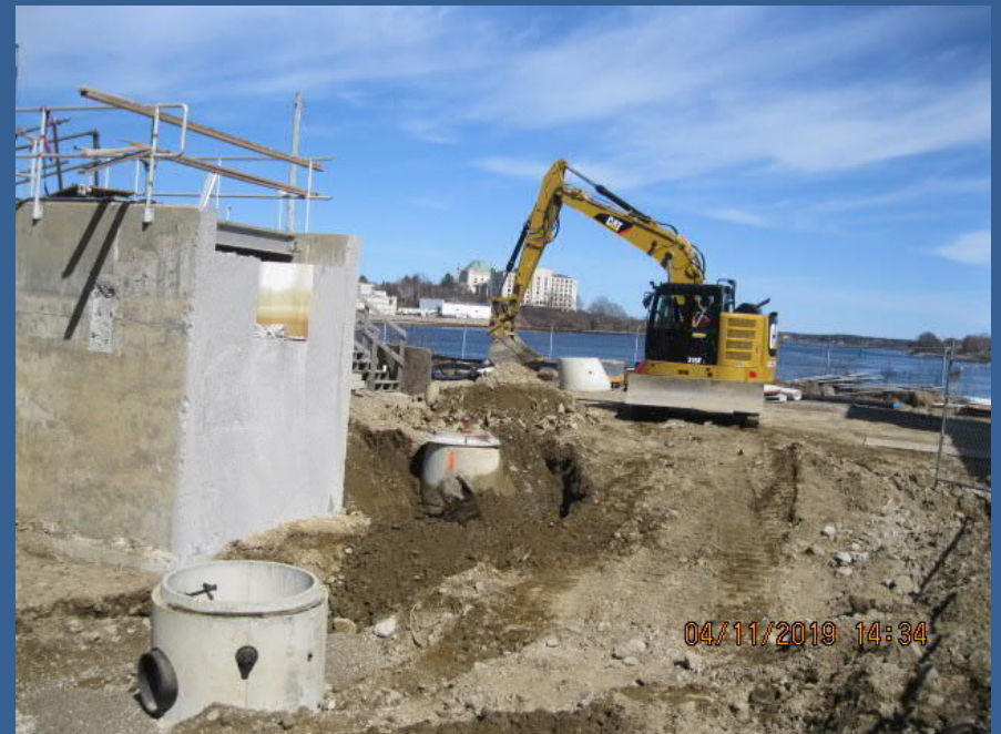
Chlorine Contact Tanks
