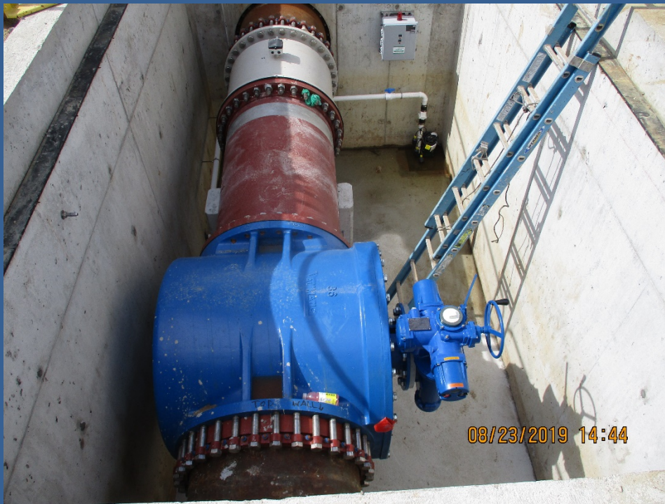
Flow Meter Vault
