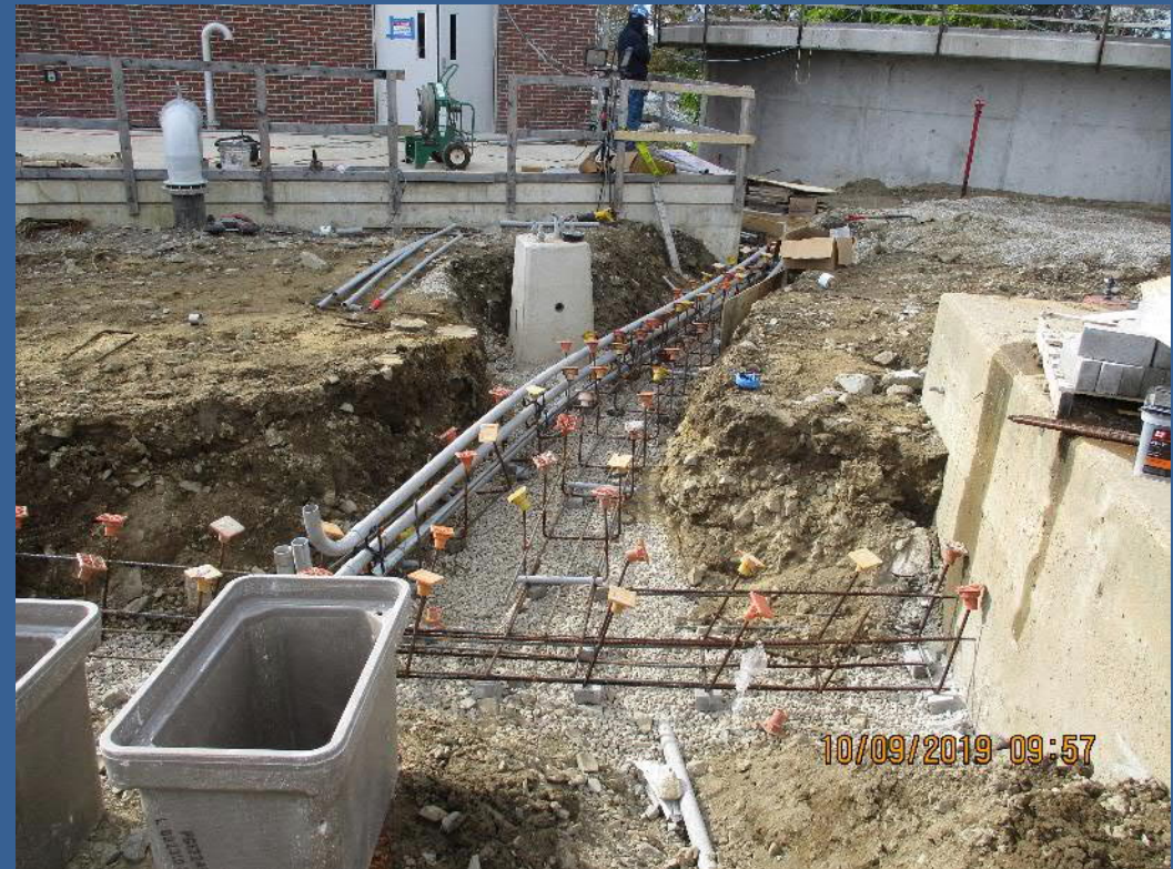
Yard Piping & Utilities
