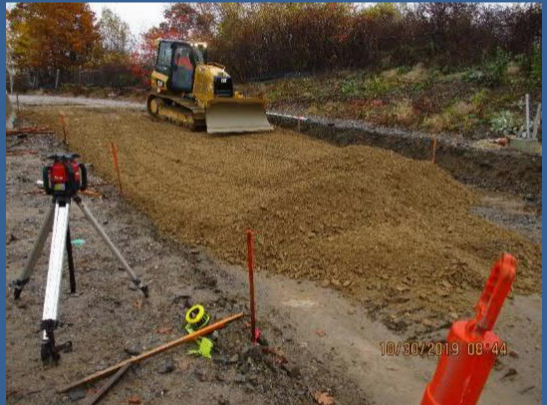
Yard Piping & Utilities
