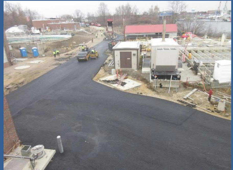
Yard Piping & Utilities
