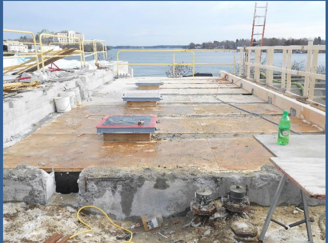
Chlorine Contact Tanks
